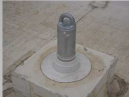
Roof mounted tieback anchor
