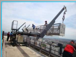
Building Maintenance Unit (BMU)
